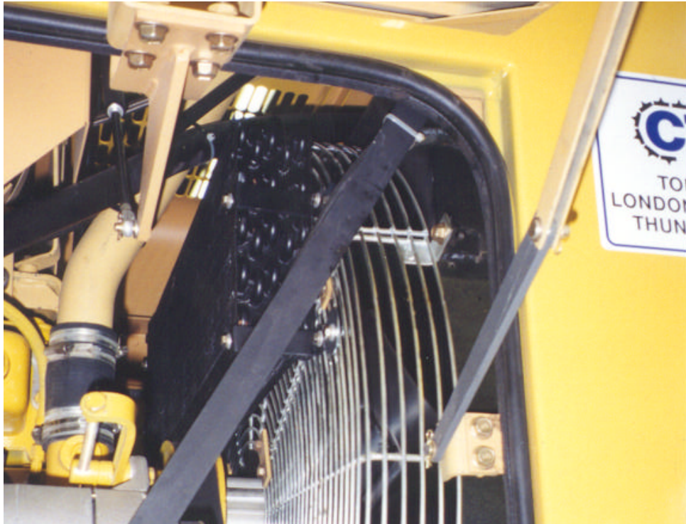
Condenser as viewed from left side.
