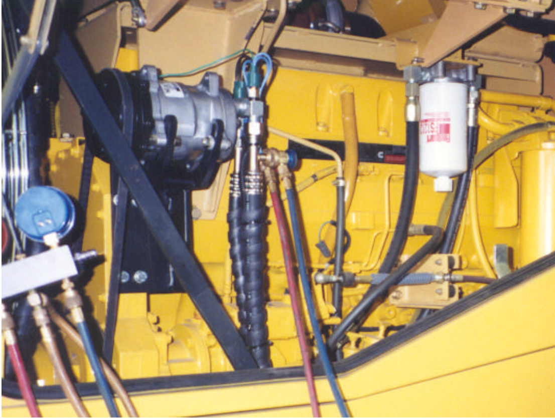
Compressor mounted and in place with drive belt and hoses.
